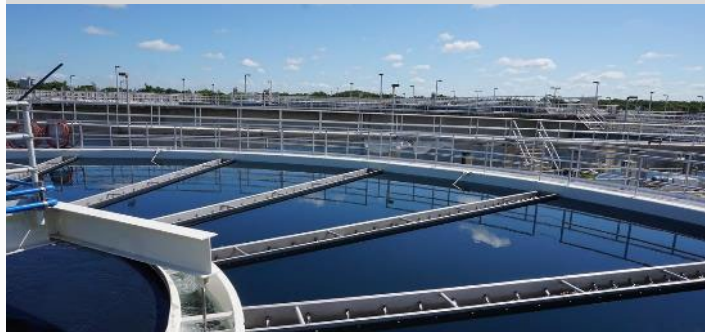
Water treatment systems
